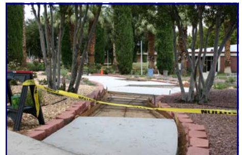
The meditation garden is getting closer to completion. Imagine a water fountain, shade structure and benches for relaxation of students, staff and faculty.
